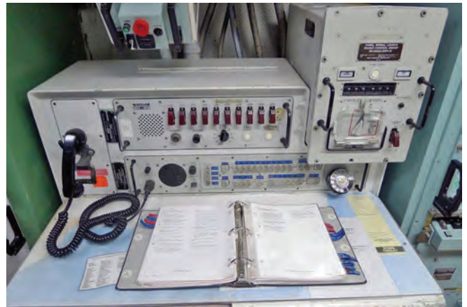
DMCCC console in D-1 LCC. This is an older design than those installed at O-0
